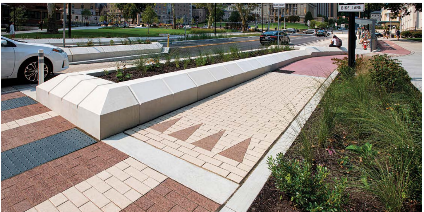
PROJECT: University of Pittsburgh - Bigelow Boulevard Complete Street, Pittsburgh, PA. DESIGN: LaQuatra Bonci Associates. PRODUCT: 4 x 12" with Series™ finish in Mocha and Smooth Premier finish in custom colors.
