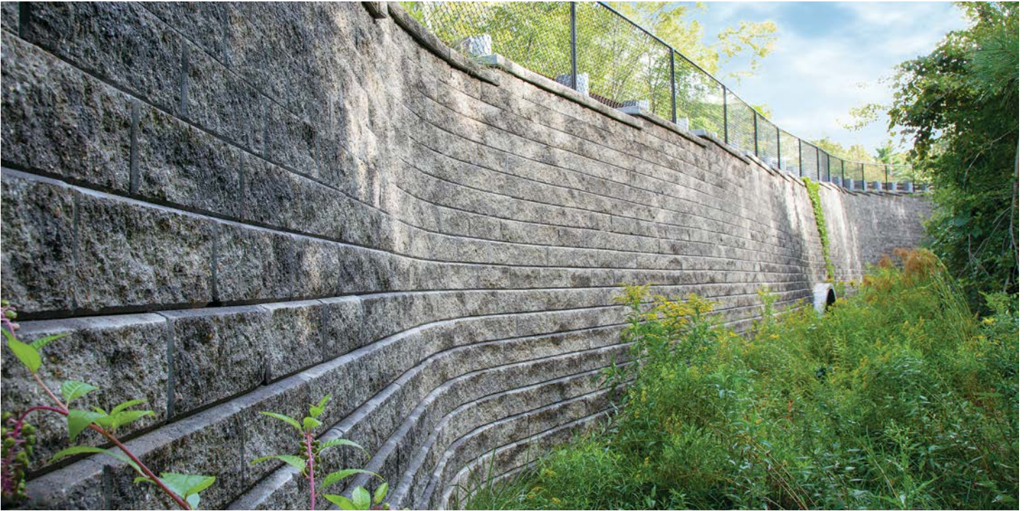
PROJECT: North Village, Douglas, MA. DESIGN: Coweaset Engineering. PRODUCT: Pisa XL / Concord Wall™ XL in Granite Blend.
